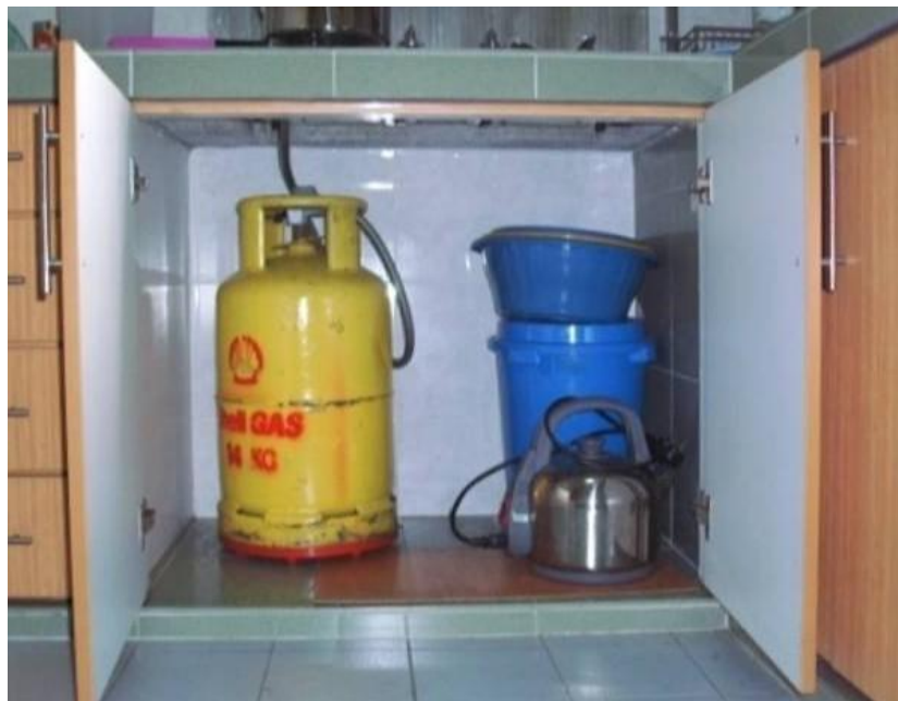
Photo 4.37. Residential propane installation, unsecured and unventilated. Skudai.
