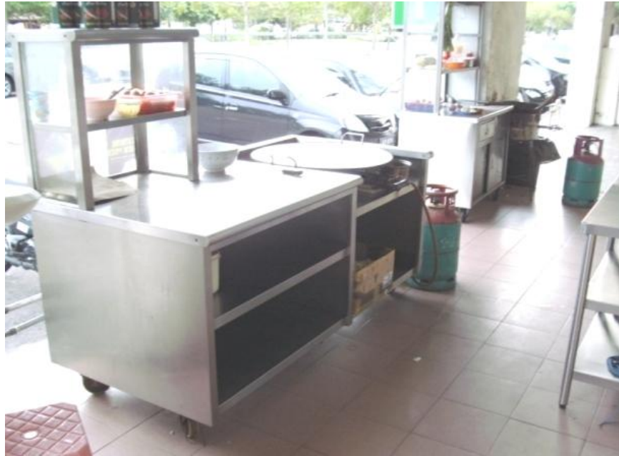
Photo 4.38. Commercial propane installation. Propane unsecured and near hot grill. Skudai.
