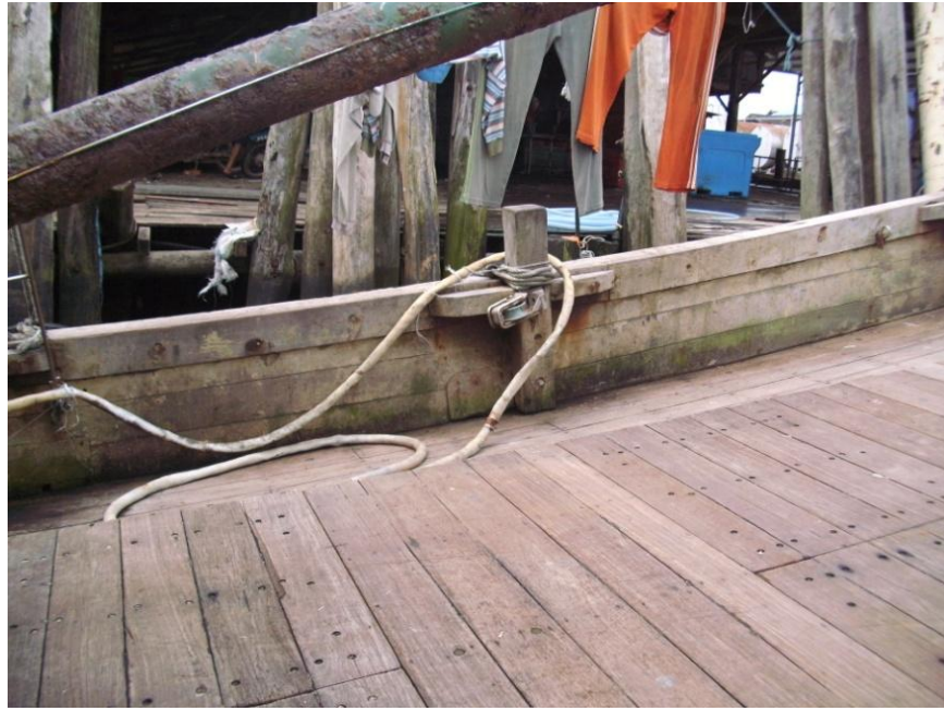
Photo 4.9. Deck usually follows sheer line which provides deck drainage. Note the misalignment with the dock and the requirement for crew to walk on the sloped surface. Endau.
