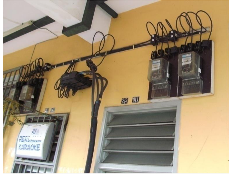
Photo 4.35. Power entrance to commercial buildings. Skudai.
