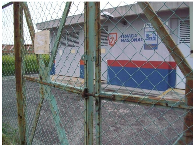
Photo 4.36. Unsecured electrical substation. Skudai.
