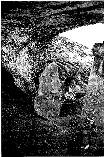
Photos 5 and 6 A poor installation - note damage to blade tips, very fouled hull surface and poor use of the space in the propeller aperture
