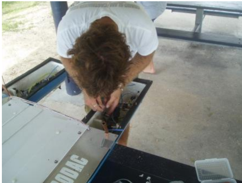
Figure 7.1: Josh attempting to re-secure the loosened motors
